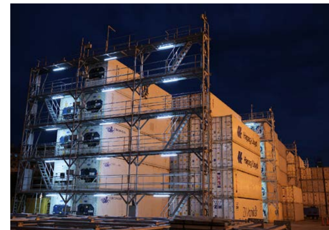
Montecon: andenes reefer / Reefer platforms
